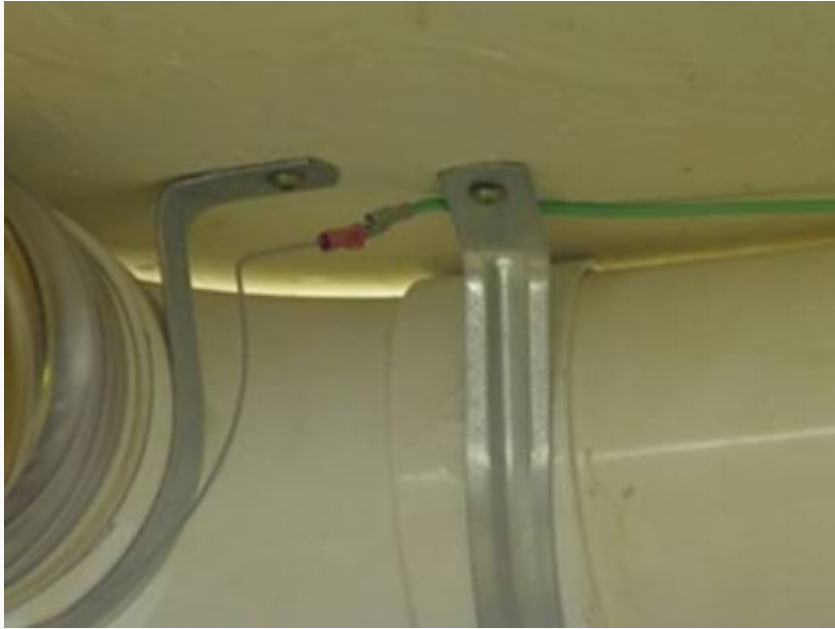
PIC# 5 Ground wire attached to the “downwind side of the dust collection hose
