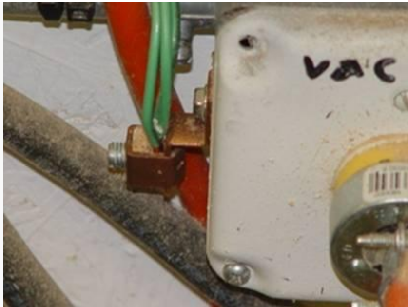
PIC# 1 Ground Lug attached to electrical box with bronze bolt thru box to #10 AWG wire inside.
